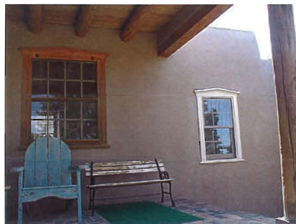
Fig. 5. Shows original wood window of living room (left) and new window in the hall of the new wing.
