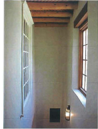
Fig. 22. Former external white window at stairs now internal and looking through repositioned former living room window
