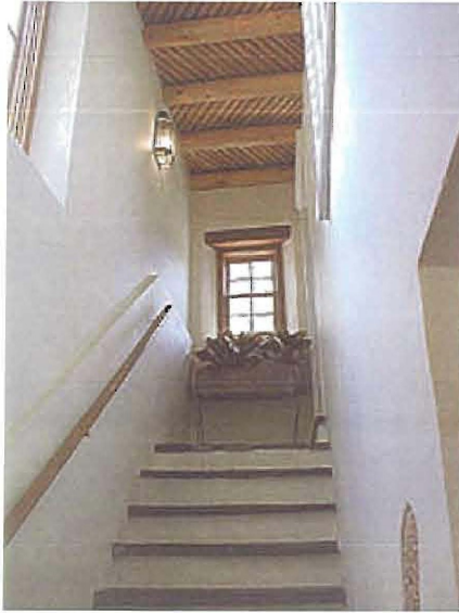
Fig. 21. View of newly enclosed stairs. Stairs are the original stone. Note the line of the former external stair railing.
